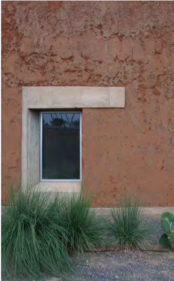
Two types of mud bricks, or adobes, were used in the construction. The lower portion has adobes made in New Mexico that possess a higher compressive strength and resistance to water. Towards the top of the wall, adobes made in nearby Ojinaga, Mexico were used that are lighter in both weight and color. The mud used in the plaster is from Van Horn and has a beautiful reddish tint.
