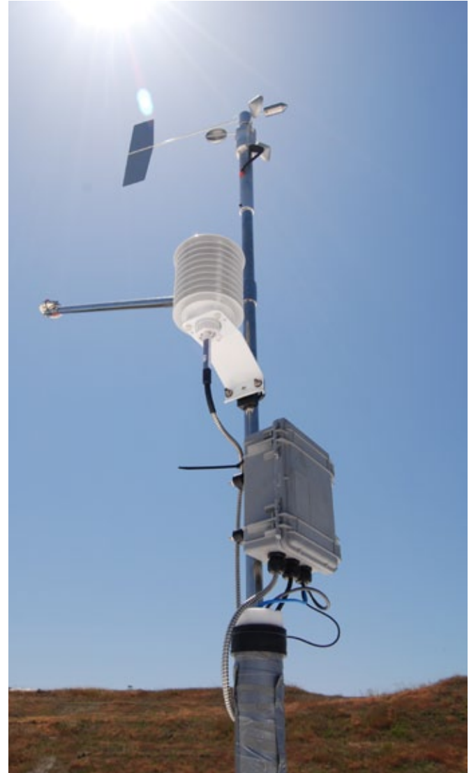
fig.0021h research-grade weatherstation installed.jpg
