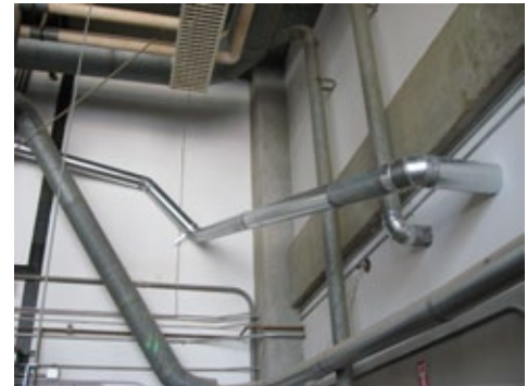
fig.0123 dust collection infrastructure.JPG
