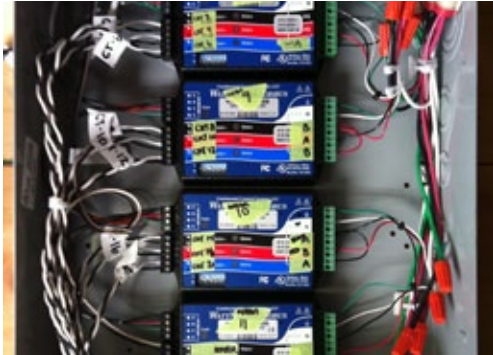
fig.0021f electrical circuit monitoring hubs.jpg
